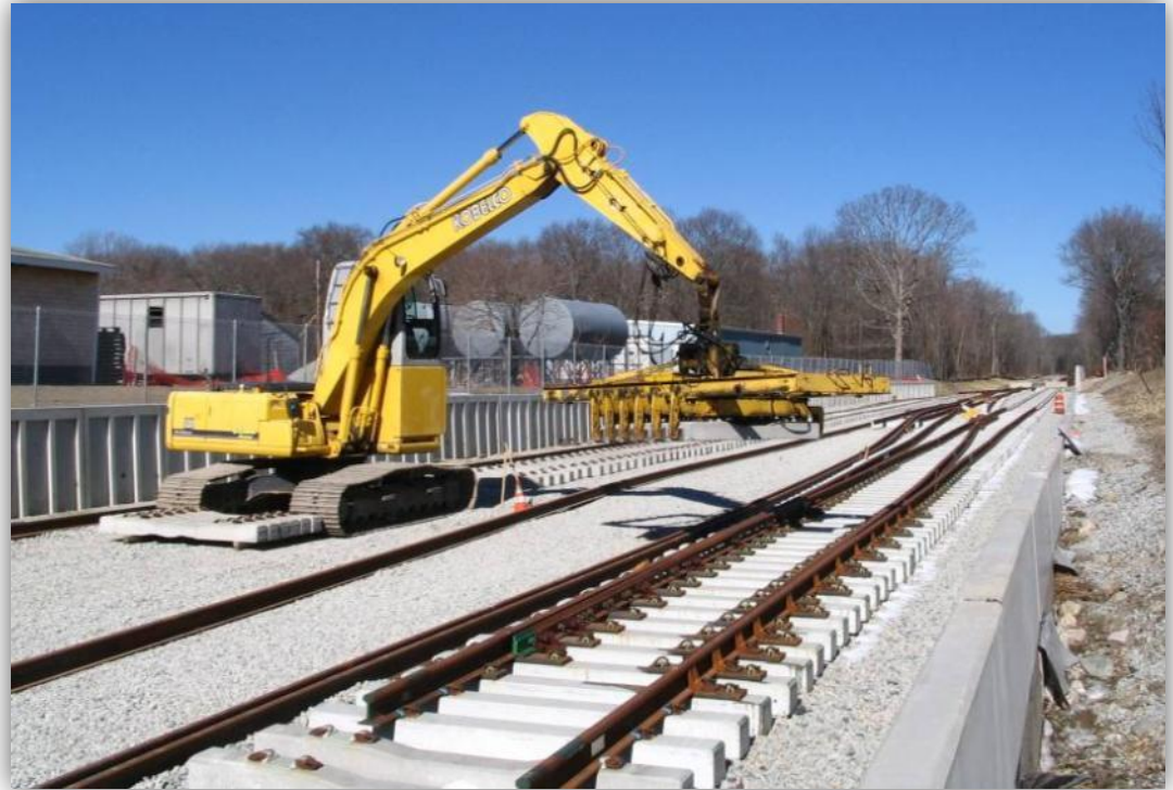
Massachusetts Bay Transportation Authority Greenbush Old Colony Commuter Rail Line Boston, Massachusetts
