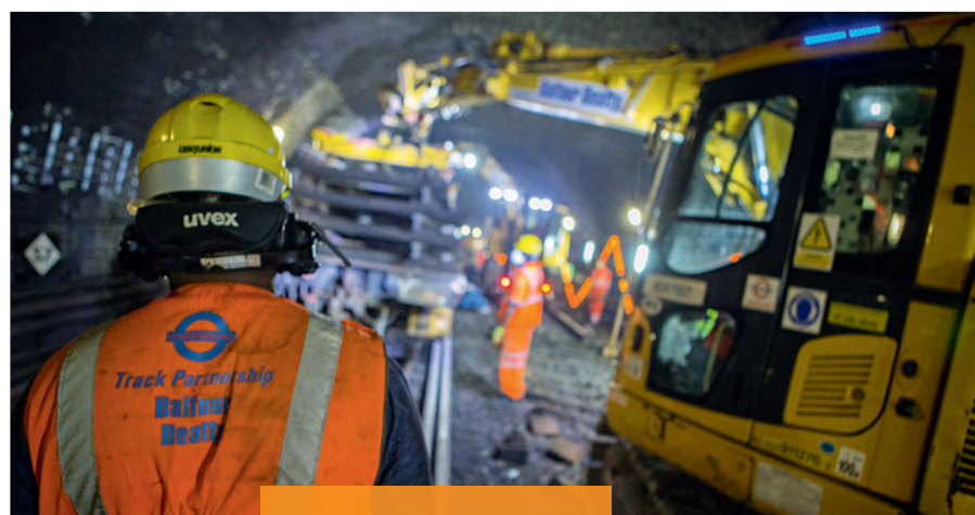
Track Partnership Balfour Beatty delivers essential track renewal work across the London Underground network.
